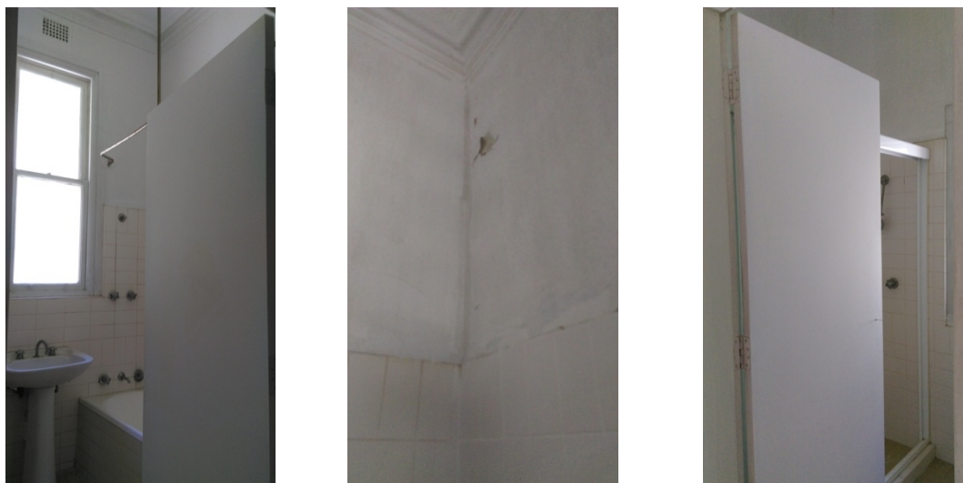
Bathrooms 3 and 4 mould damage in walls
