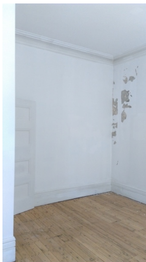
Room 11 falling damp from external roof failure
