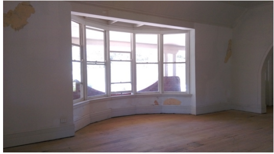
Room 1 conservation issues
