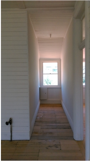
Hall 5 Sagging ceiling
