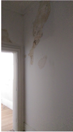
Room 10a (Cool Room Davies) Poor condition
