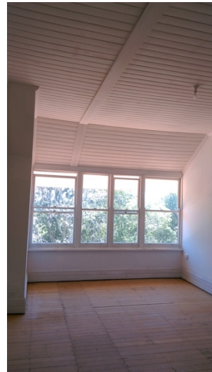
Room 18 sagging ceiling
